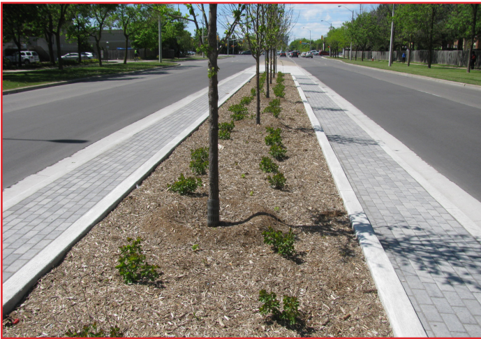
Stormwater management in the median underground bioretention.
